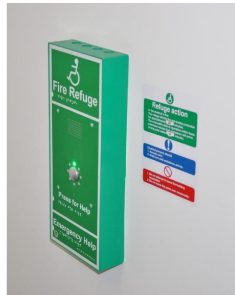
Figure 30: Photo of a Refuge Communication System, by Baldwin Boxall
