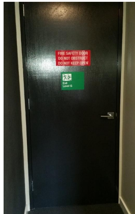
Figure 40: Photo of an Accessible Exit Sign (Installed on a Fire Door)
