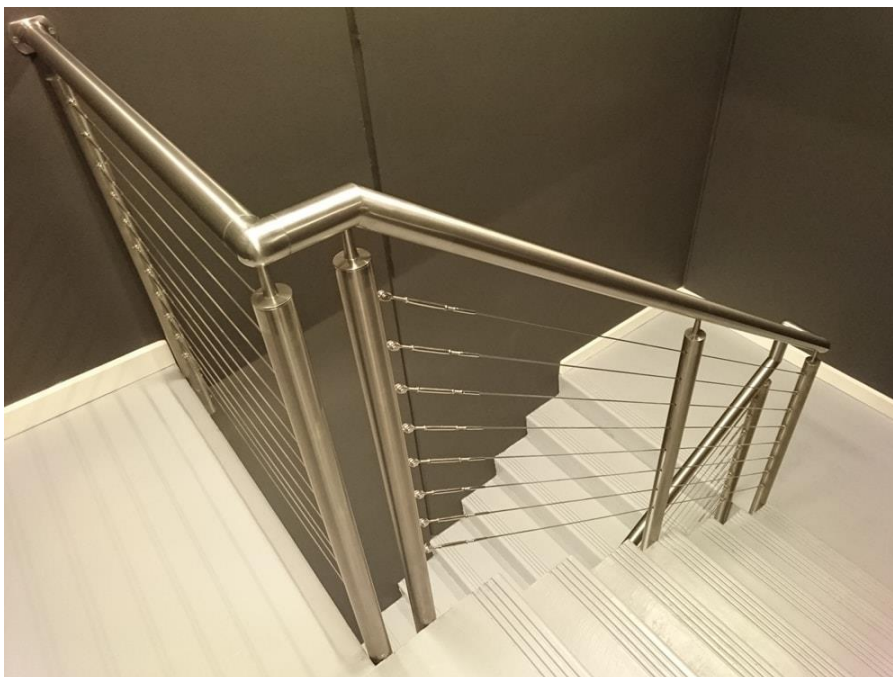
Figure 24: Photo of Single Internal Handrail in Exit Stair
