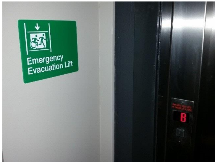
Figure 15: Photo of an Emergency Evacuation Lift Sign on Wall
