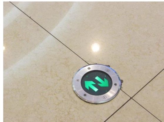
Figure 33: Photo of Directional Exit Floor Mounted Sign in China
